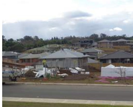
Figure 20: New detached homes under construction with insulation material in the foreground. Photo: from the project image bank, collected by the research team during site visits.
