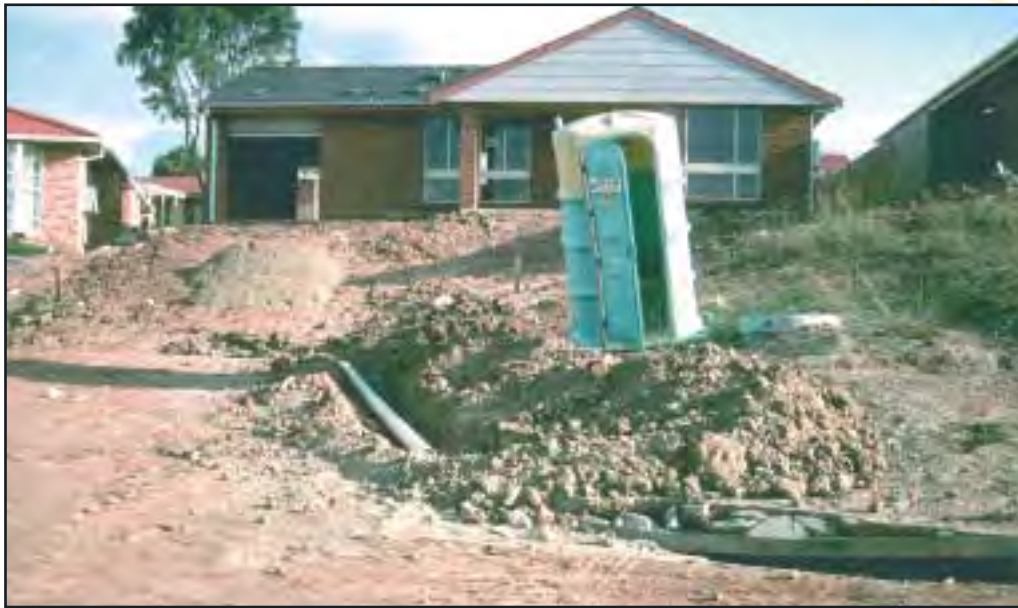
Figure 6.1 Sediment deposition below a housing construction site. As a result, the bitumen road and kerb and gutter are barely distinguishable – only a drop inlet is clearly visible
