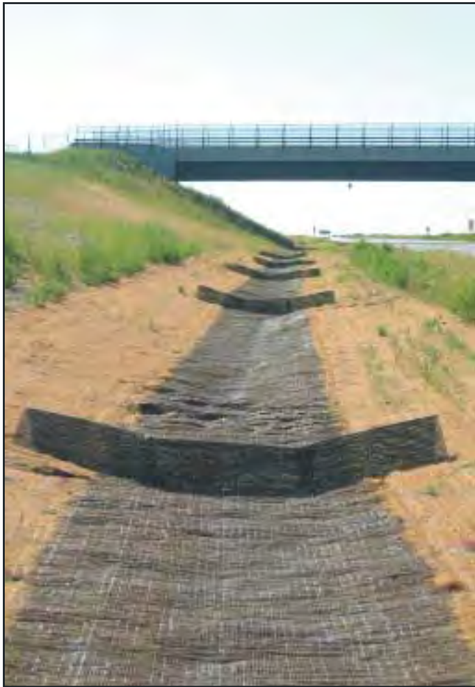
Figure 5.3(b) Alternate check dam system. Where products like these are used, they should be installed with an appropriate erosion control blanket below them and covering at least 0.7 metres each side (c.f. SD 5-4)
