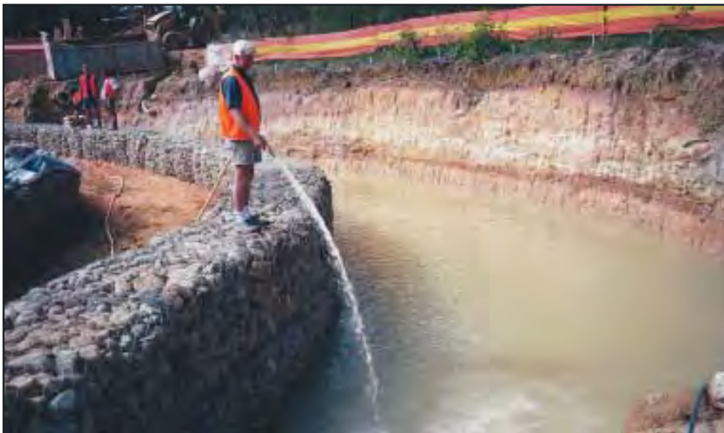
Figure E2. Poor gypsum application technique.
