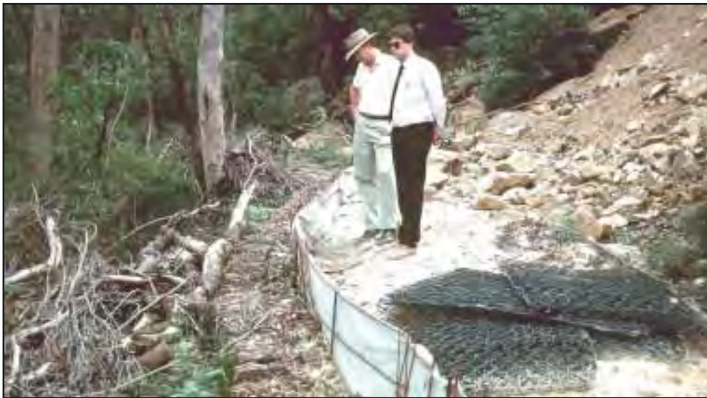
Figure 6.9 Sediment fence constructed below a fill batter – the sediment pollution is the result of a recent storm event
