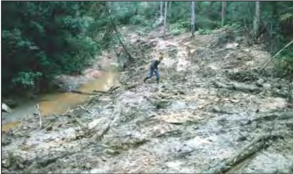
Figure 7.4 Lack of site stabilisation of a drainage line following installation of services
