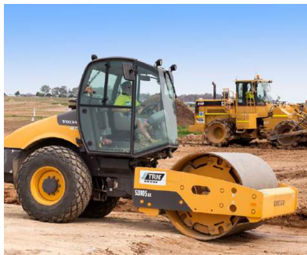
Civil works construction at the Oran Park Town community in Oran Park.
