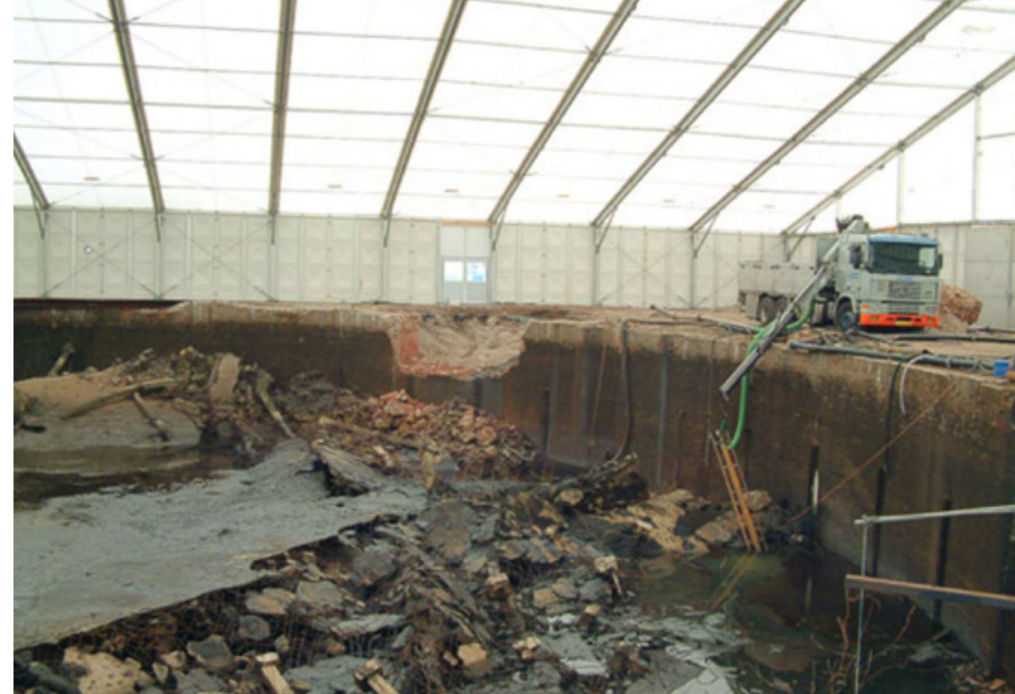
BEFORE: Gas holder during clean up in 2000 with a tent constructed over it to trap hazardous gases (Project Westergasfabriek, 2018)
