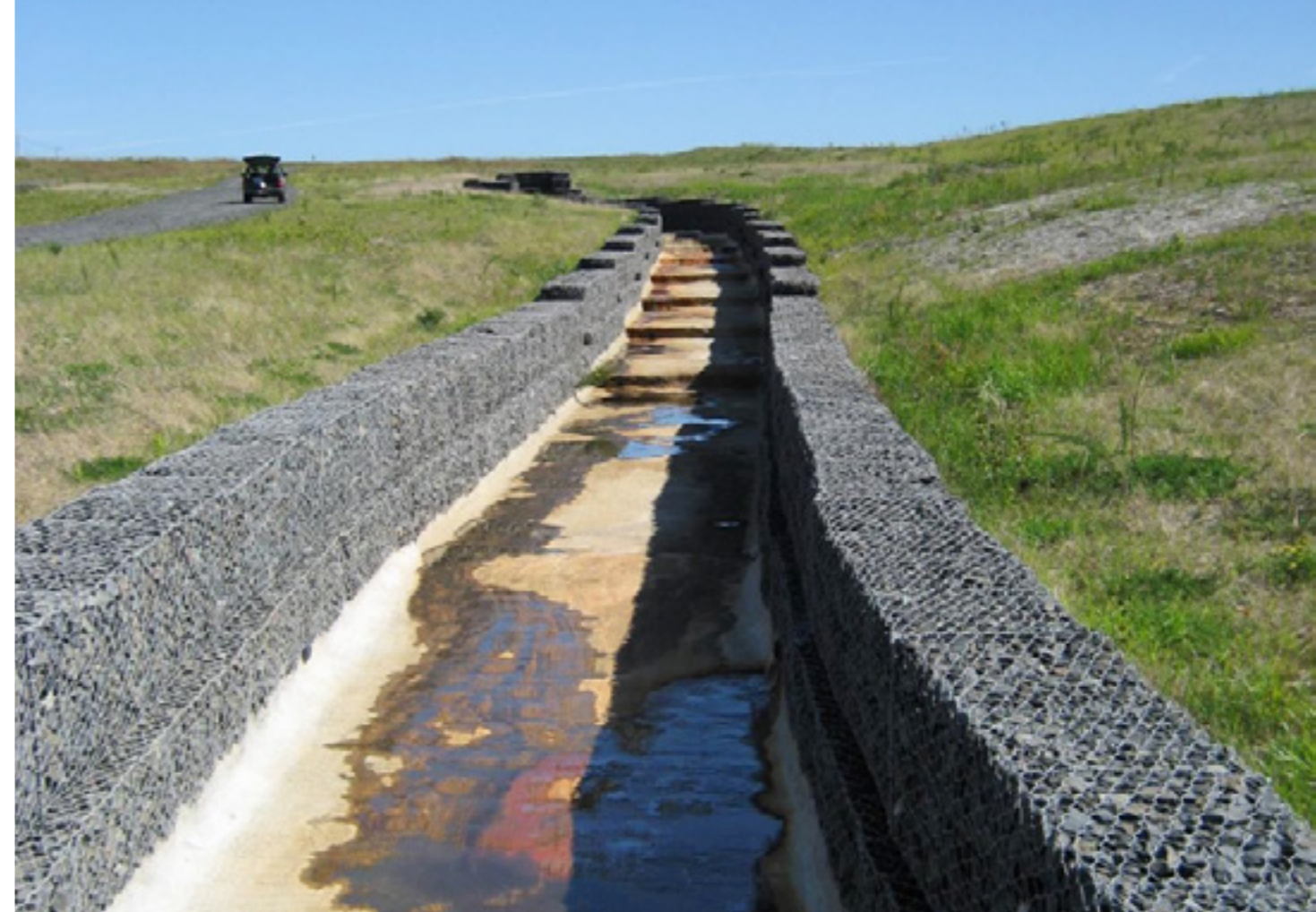
Access stormwater that drains through the cap is collected in a network of swales, channels and downchutes and then stored in detention basins at the bases of the hills. Gabion retaining walls support the soil matrix. Image taken from Freshkills Park Instagram account, 2017
