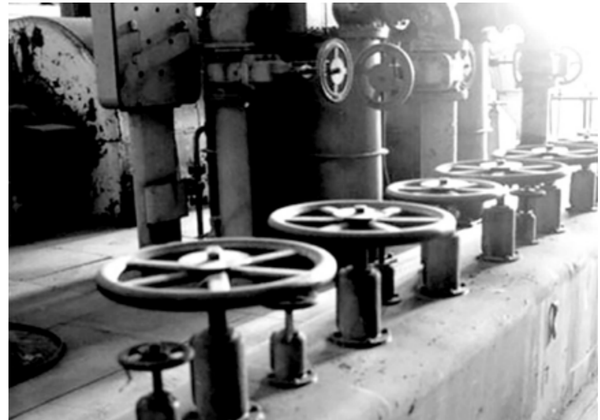
Parsons turbine and pumps, WBPS.
