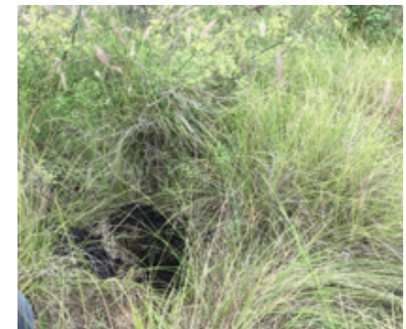
Test hole 7. Dense root system due to grasses. Large poly pipe beneath found to be disconnected.
